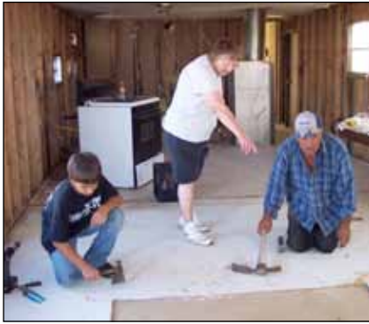
To prepare the mobile home for use as a temporary sanctuary and office, old flooring and walls were removed and replaced with new.
